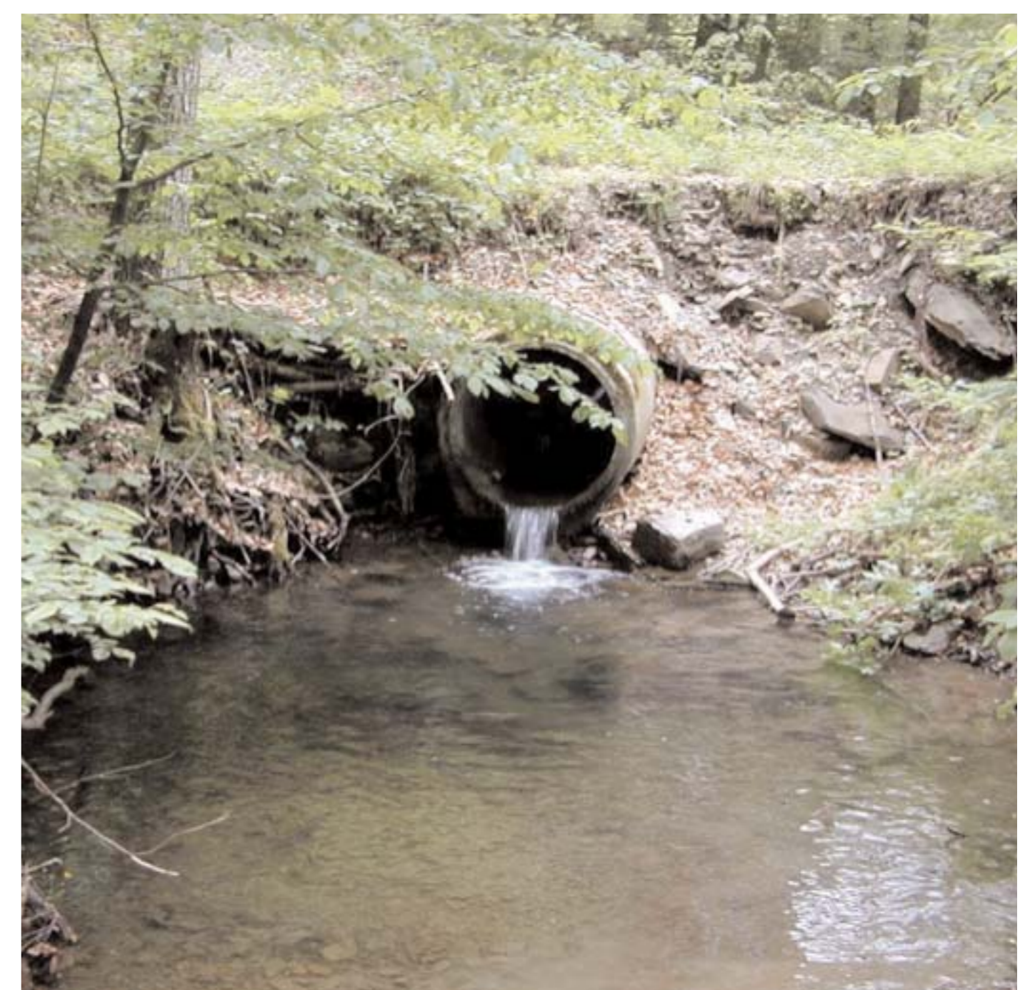
Fig.5: One of the pipes interrupting the Münichbach creek's lower course and obviously inhibiting contacts between the upper course stone crayfish and infectious signal crayfish. G. Pfundner
